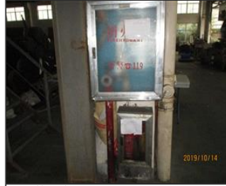
Photo of fire safety equipment Fire hydrant Fire extinguishers.JPG
