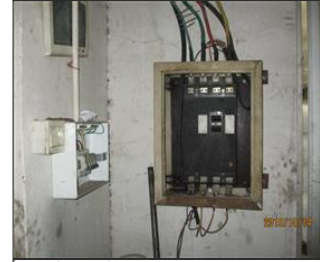
Photo of non-conformity 7.13 Electric boxes had no external covers.JPG
